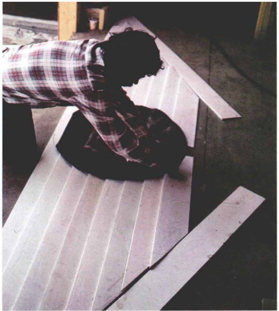
To fit clapboards around a round window, the clapboards are laid out on the ground and a pattern of the window, made of building felt, is traced onto them.
